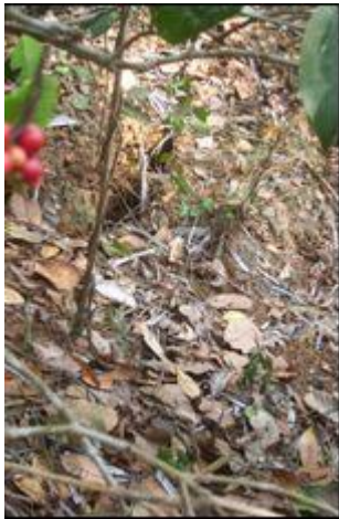
Photo10:Crown cracks observed in between Sasanwad Slide no-2 & slide no-3.
