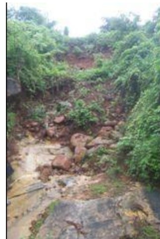
Photo 4: A view of top portion of Sasanwad slide no-2.
