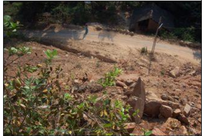
Photo 16: Survey work in progress at the top of Sasanwad slide no-3 with lush vegetation of cashew plantation all around.
