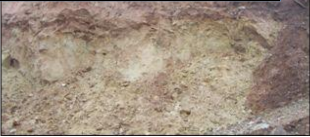
Photo 7: Highly wetahered dyke in Sasanwad slide no-3.
