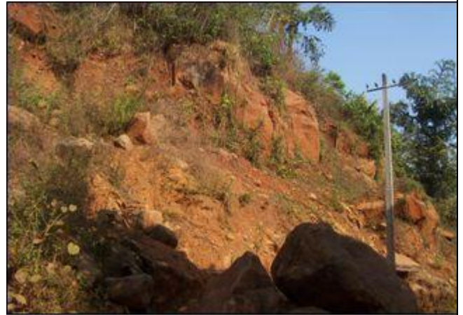
Photo 14: View of road from the crown part of Sasanwad slide no-3.
